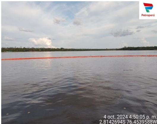
Picture 5. Installation of containment barriers on the Pastaza River (Installed on October 03, 2024, and taken on October 04, 2024).
