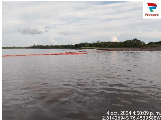
Picture 6. Installation of containment barriers on the Pastaza River (Installed on October 03, 2024, and taken on October 04, 2024).
